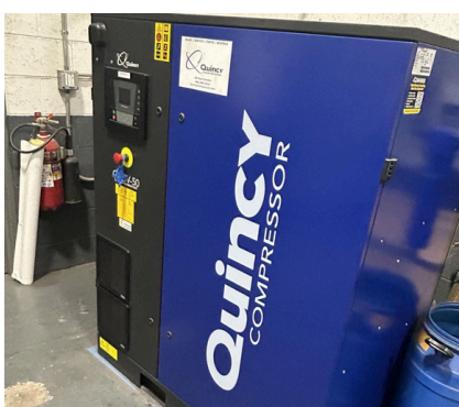
Air Compressors and Dryers - Ingersoll-Rand + Quincy
